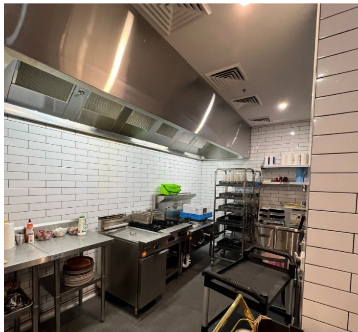
Figure 40 Industrial kitchen at 94 Hay Street.
